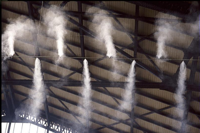
Direct evaporative Cooling system - Marseille Saint-Charles station, France.
