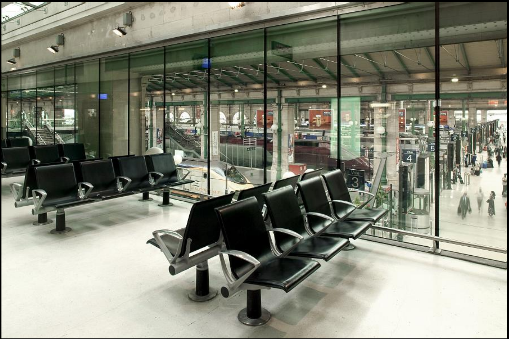
Heating system integrated into the glazing – Paris-Nord station
